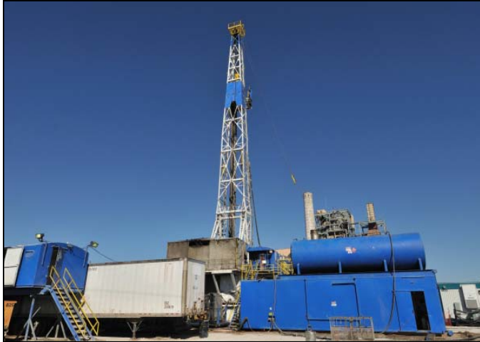
Drilling of New Class I Disposal Well at Mid Kansas Electric Cooperative in Dodge City, Kansas
