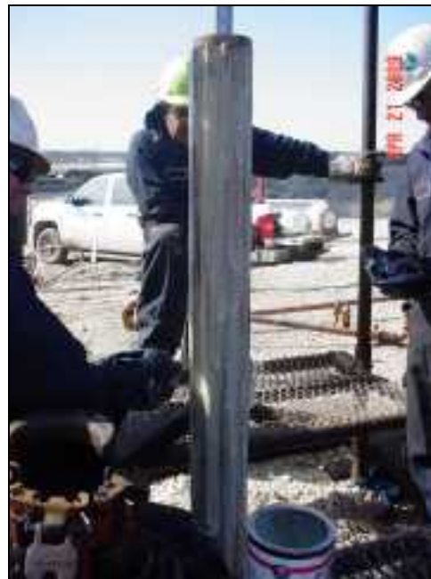
Applying Epoxy to Casing Patch used to Repair Longstring Casing in Class I Well
